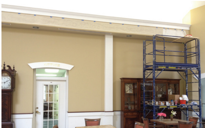
The tracing paper template was taped to the soffit with Saral Transfer Paper underneath.
