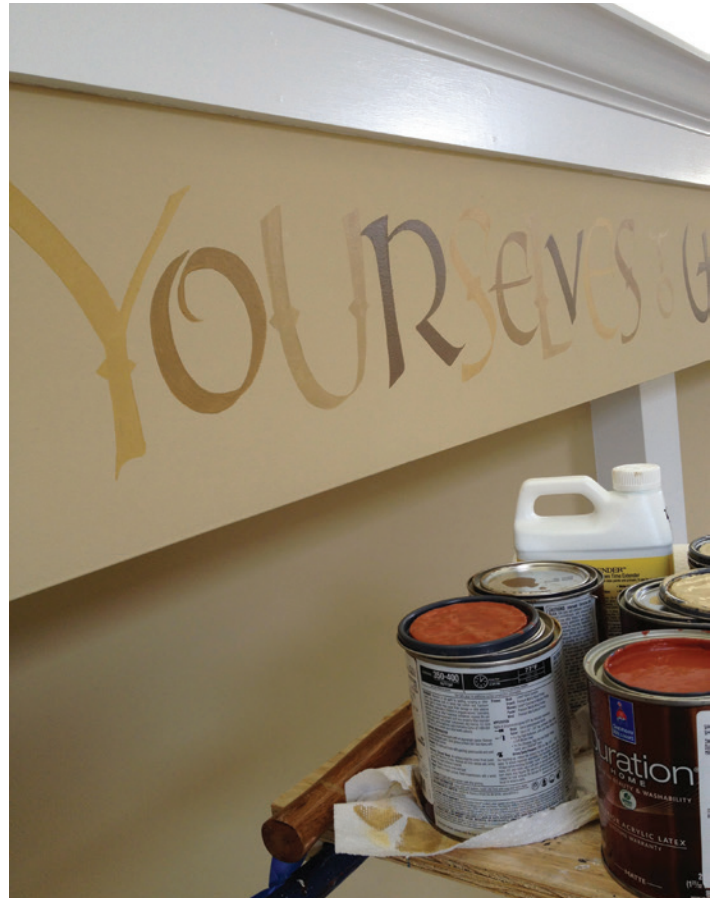
Interior house paint was used for the letters. It was thinned with extender to get a decent flow.
